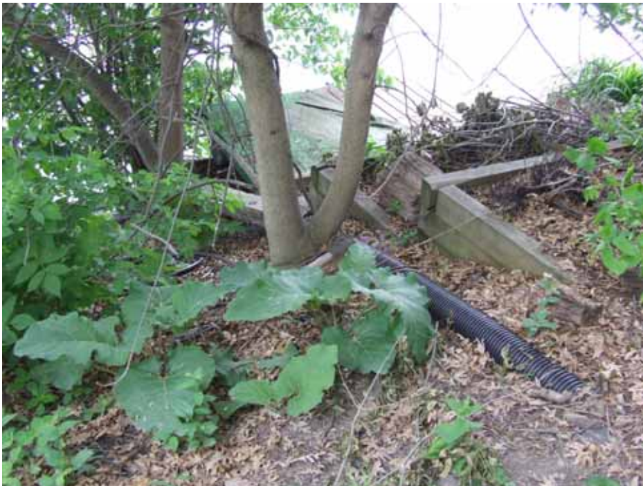
ID54: 3212/3210 West Owasso Blvd. – 8” flexible plastic pipe
