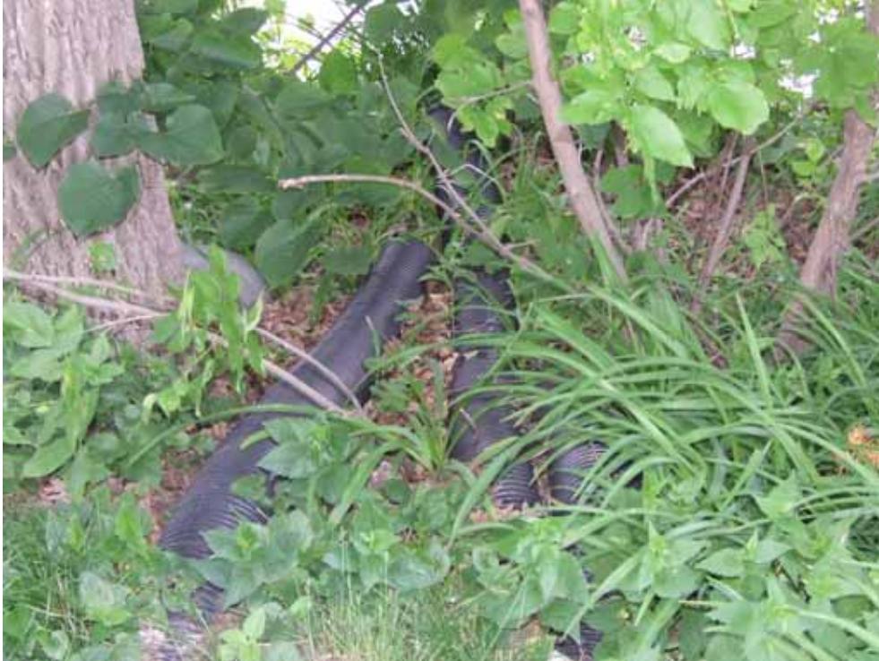
ID47: 3216/3212 West Owasso Blvd. – 3 – 8” flexible plastic pipes
