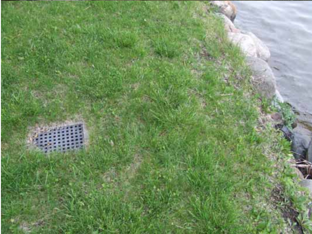
ID49: 3198 West Owasso Blvd. – 2 – 4” flexible plastic pipes with some inlets in the yard
