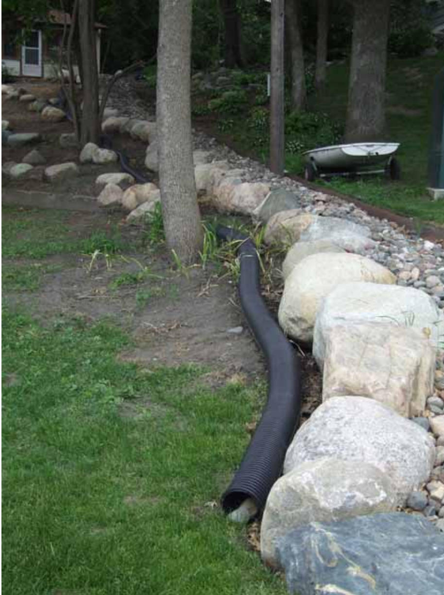
ID51: 3192 West Owasso Blvd. – 8” flexible plastic pipe
