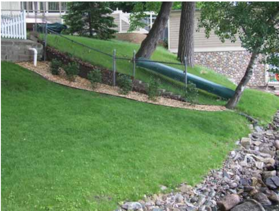
ID42: 458 West Horseshoe Drive – 4” PVC drains into 4” flexible plastic
