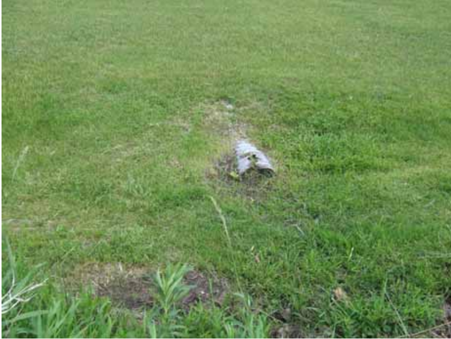
ID50: 6-6-7 004 – Drain from Owasso Blvd. N near 291. 12” CMP, plugged.
