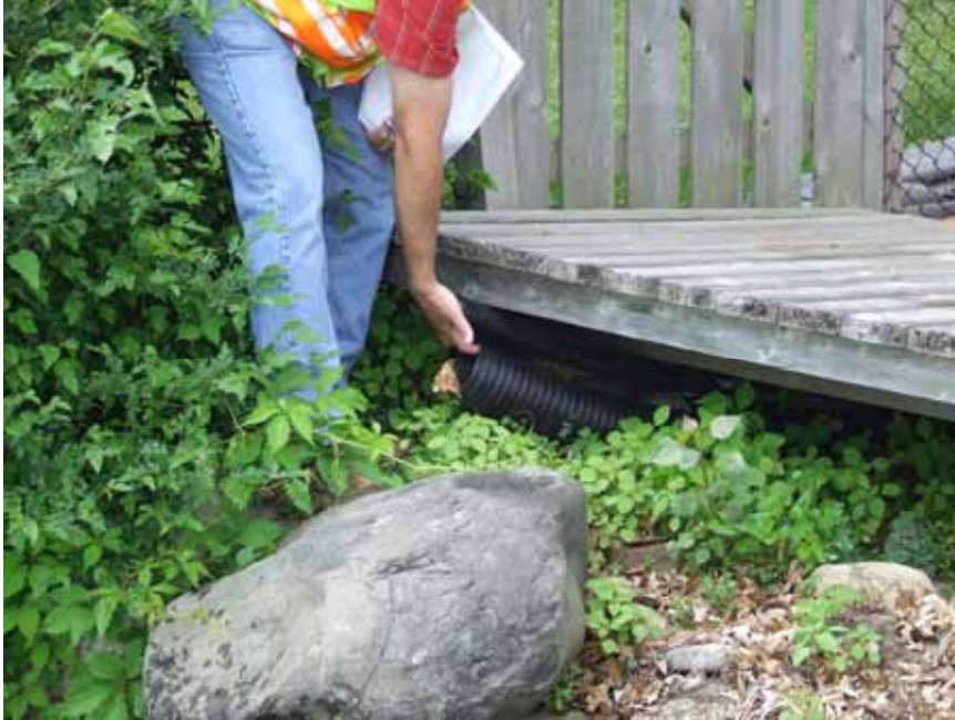
ID44: 3288 Owasso Heights Road – 4” flexible plastic pipe and 2” PVC
