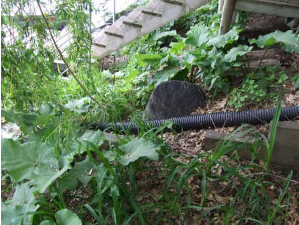
ID48: 3210/3206 West Owasso Blvd. – 4” flexible plastic pipe
