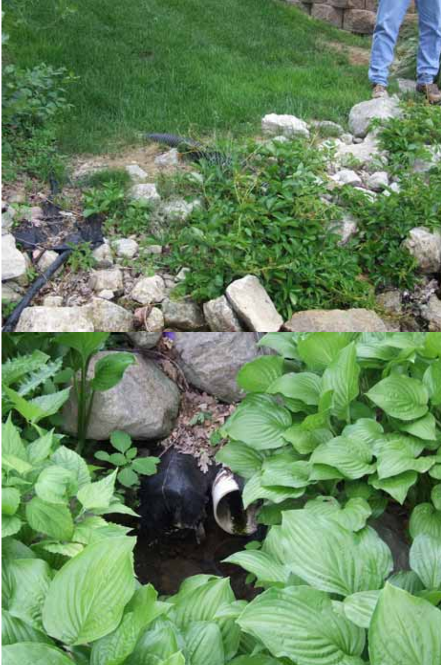
ID43: 3320 Owasso Heights Road – 2 – 8” PVC pipes and 1 – 4” flexible plastic pipe
