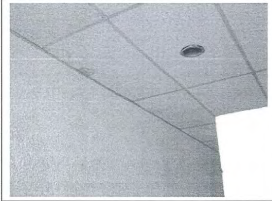
Facing: Up View of: Water stained ceiling tiles in stairwell to basement
